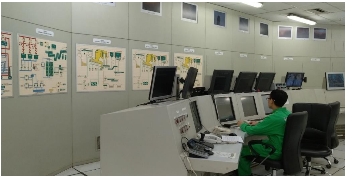
Figure 5. The Central Control Room of the Incineration Center (Image Source: Photographed by the Author)
