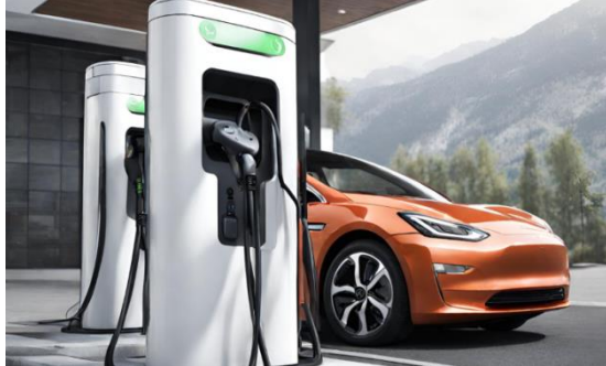
Figure 2: Charging station in Commercial building.
