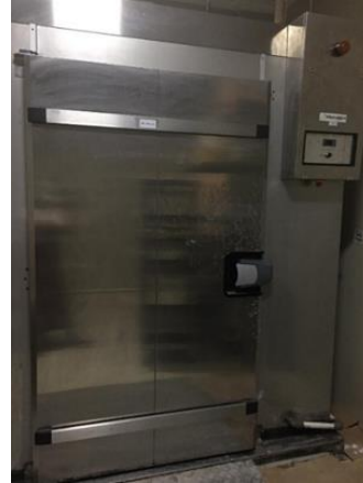
Figure 2. Blast Freezer Machine
