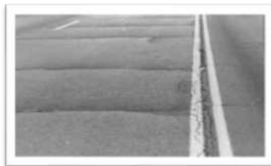
Gambar 7. Retak Refleksi ( Reflection Crack ) Sumber: Bina Marga No.03/MN/B/1983
