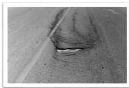
Gambar 9. Retak Slip (Slippage Crack) Sumber: Bina Marga No.03/MN/B/1983
