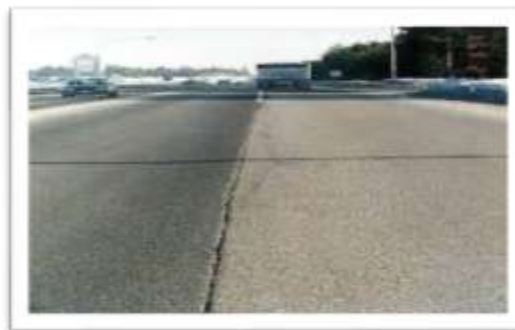
Gambar 5. Retak Sambungan Lajur (Lane Joint Crack) Sumber: Bina Marga No.03/MN/B/1983
