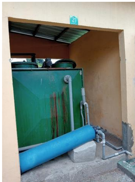
Figure 3. Waste Water Treatment Installation Equipment (IPAL)
