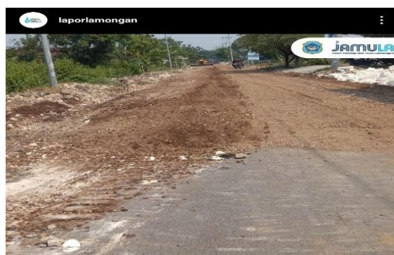
Figure 4. Government Response to Reported Road Repairs
