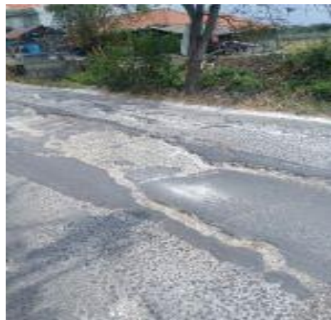
Figure 1. Severely Damaged Alternative Road between Lamongan and Gresik
