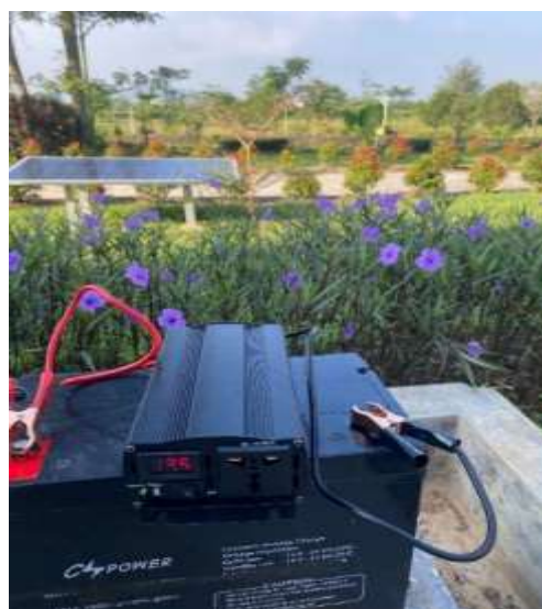
Figure 3. Battery and Inverter
